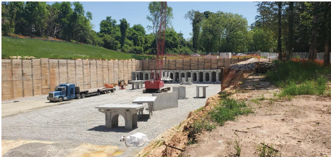
Figure 12. Construction of the larger of the two pre-cast concrete vault systems, BMP 6.
