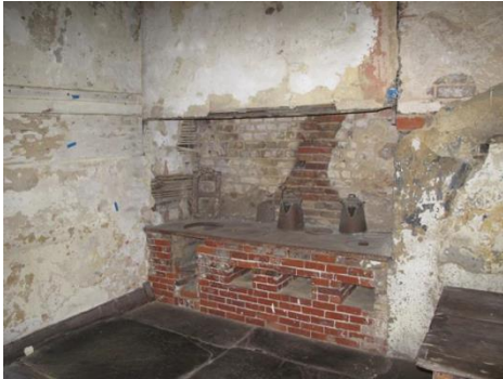
4.34 K101-II-5. East wall, plaster above later installations of stew stove, 1858 plaster on circular sawn lath, for comparative dating Visible Light 100X
