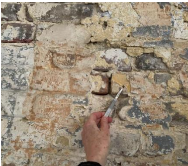
4.59 K-4. Kitchen, east wall, washes and plaster on filled in door Visible Light 40X
