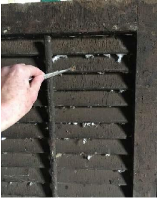
4.80 9. Detached louvered shutter, on interior side Visible Light 100X
